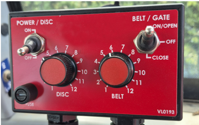
In-cab controls for belt, spinners, and hydraulic flow gate
